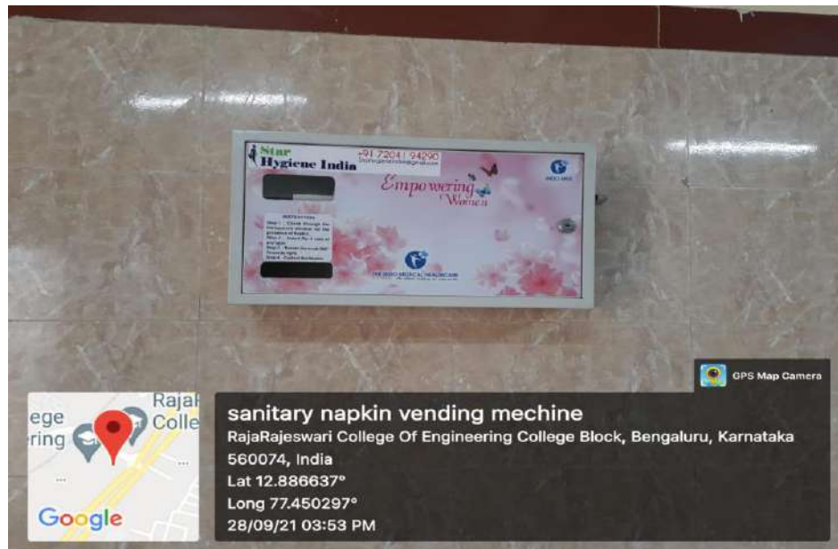
Photo.16: Sanitary napkin vending machine inside the wash room
