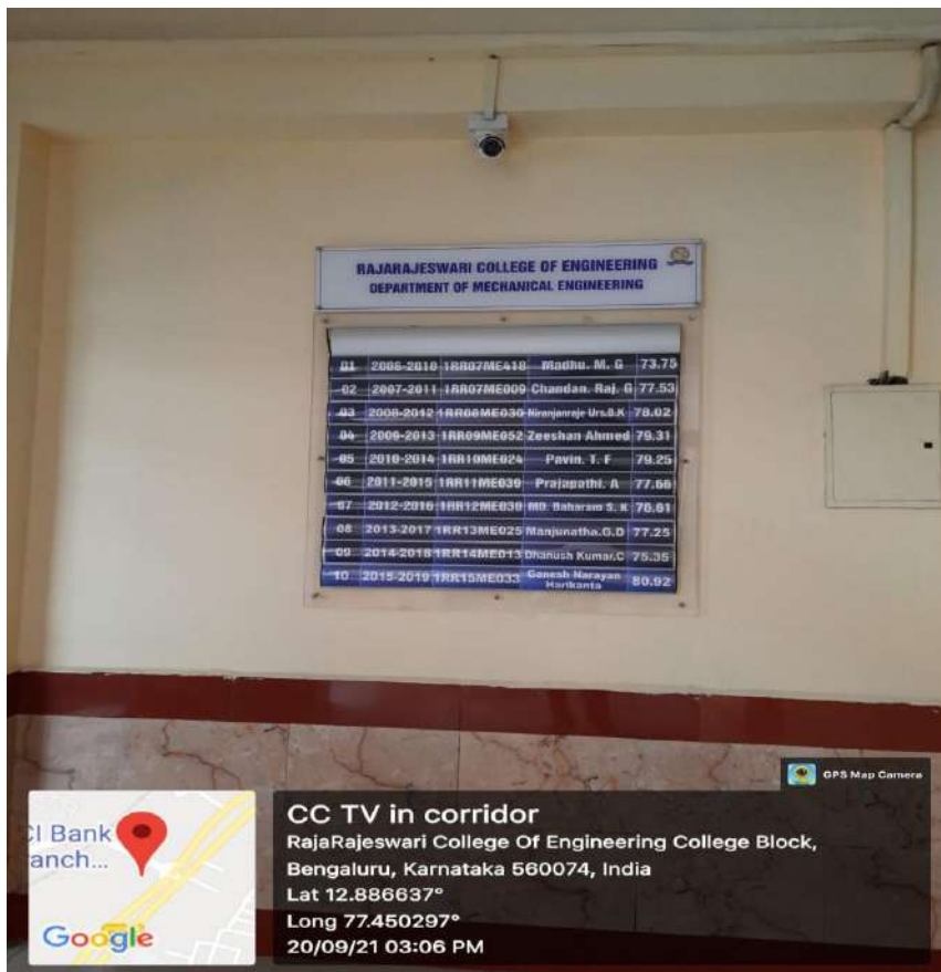
Photo.2: CCTV Camera in corridor
