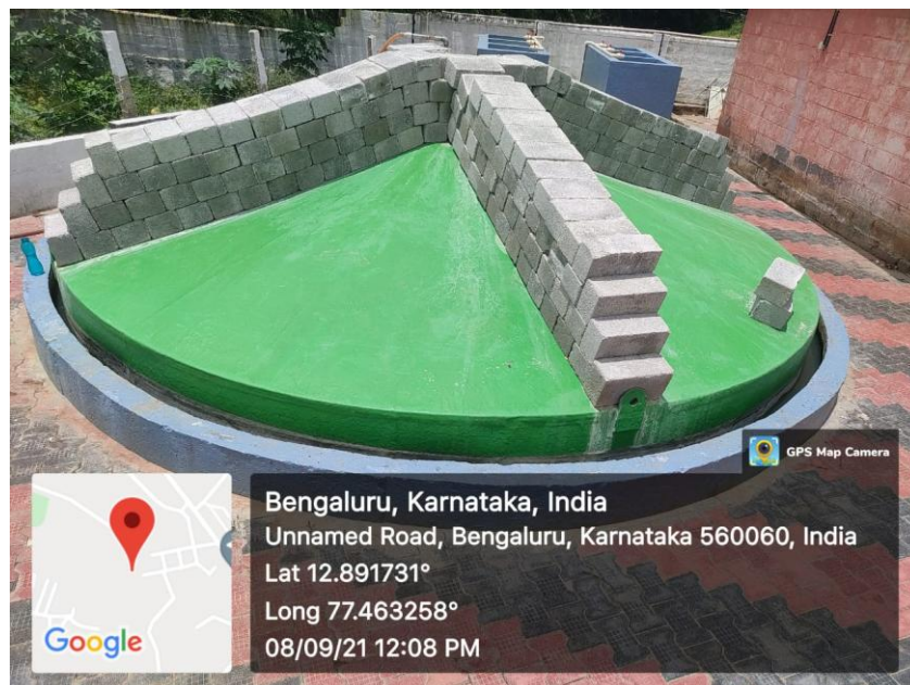
Photo.3: Centralized Biogas plant facility at RajaRajeswari Medical College and Hospital.
