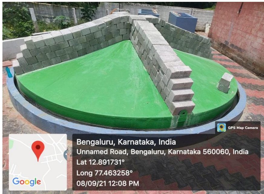
Photo.2: Centralized Bio-gas plant at RajaRajeswari Medical College and Hospital (RRMCH)
