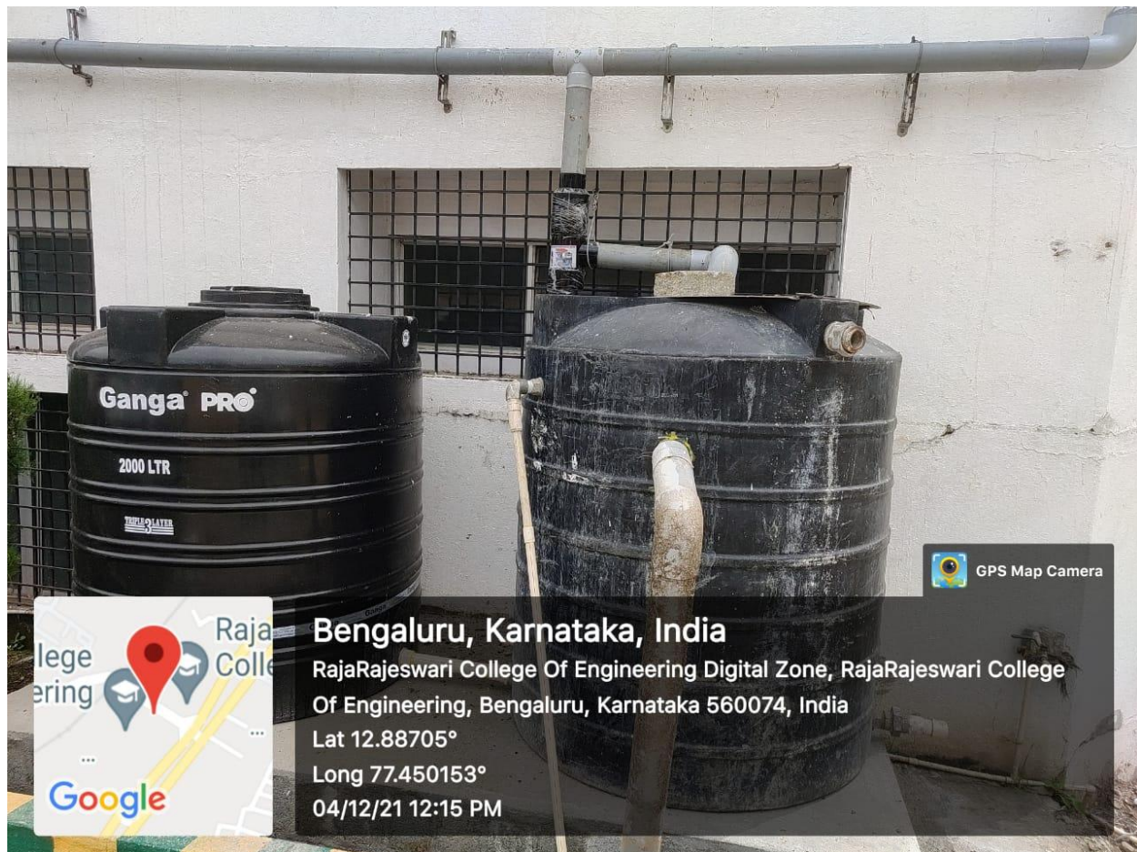
Photo.1: Rain water harvesting facility inside the campus
