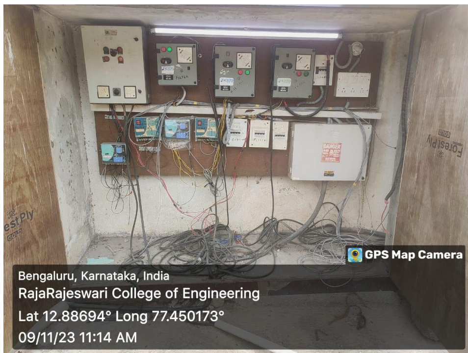
Photo.5: Sensor based 82.5 KVA Generator set systems in RajaRajeswari College of Engineering
