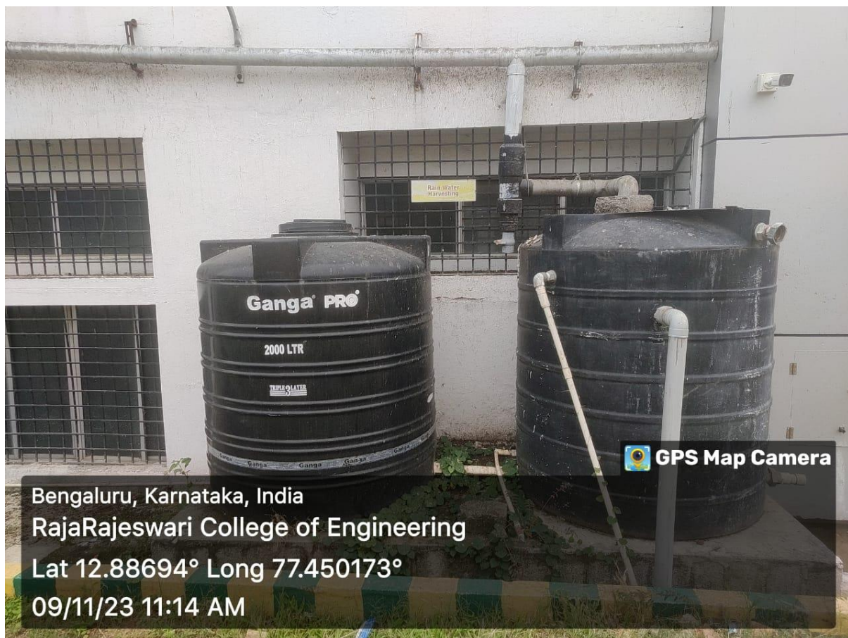
Photo.1: Rain water harvesting facility inside the campus
