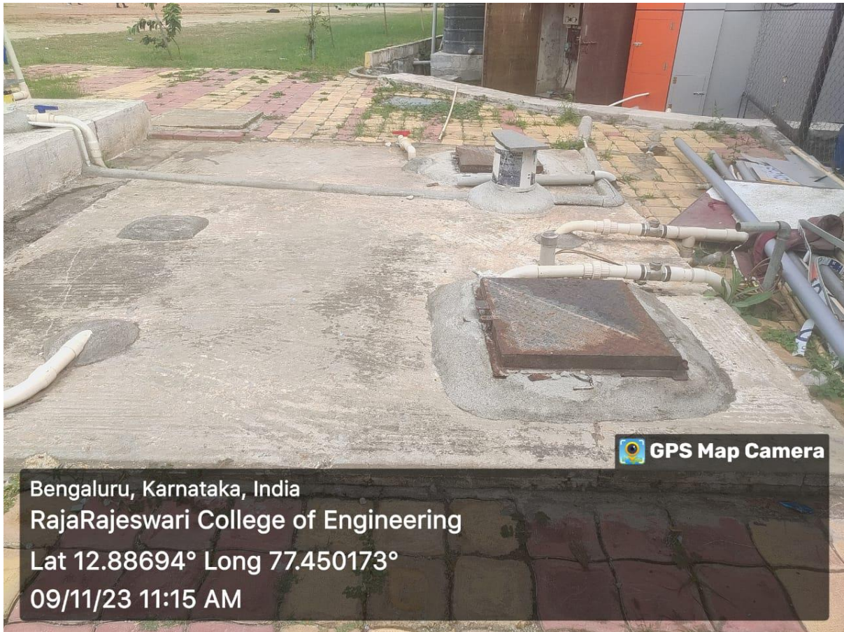
Photo.3: Water storage tanks in the campus
