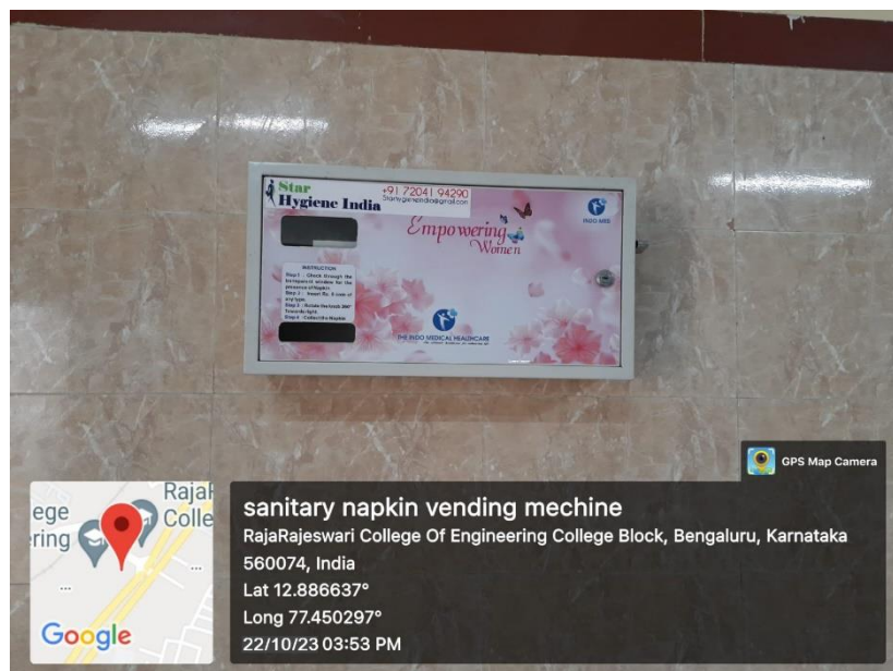
Photo.14: Sanitary napkin vending machine inside the wash room
