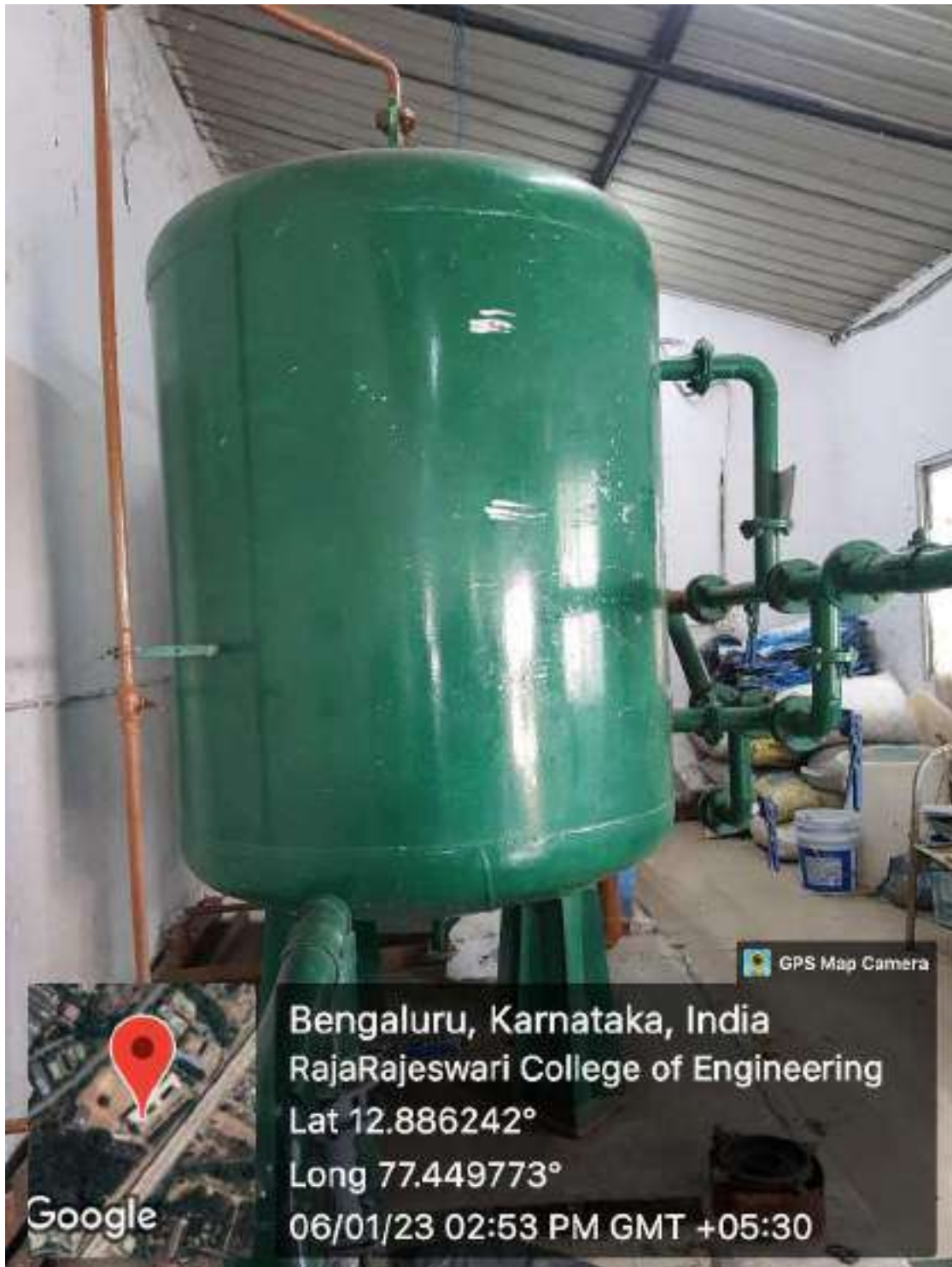
Sewage Treatment Plant facility at RRMCH
