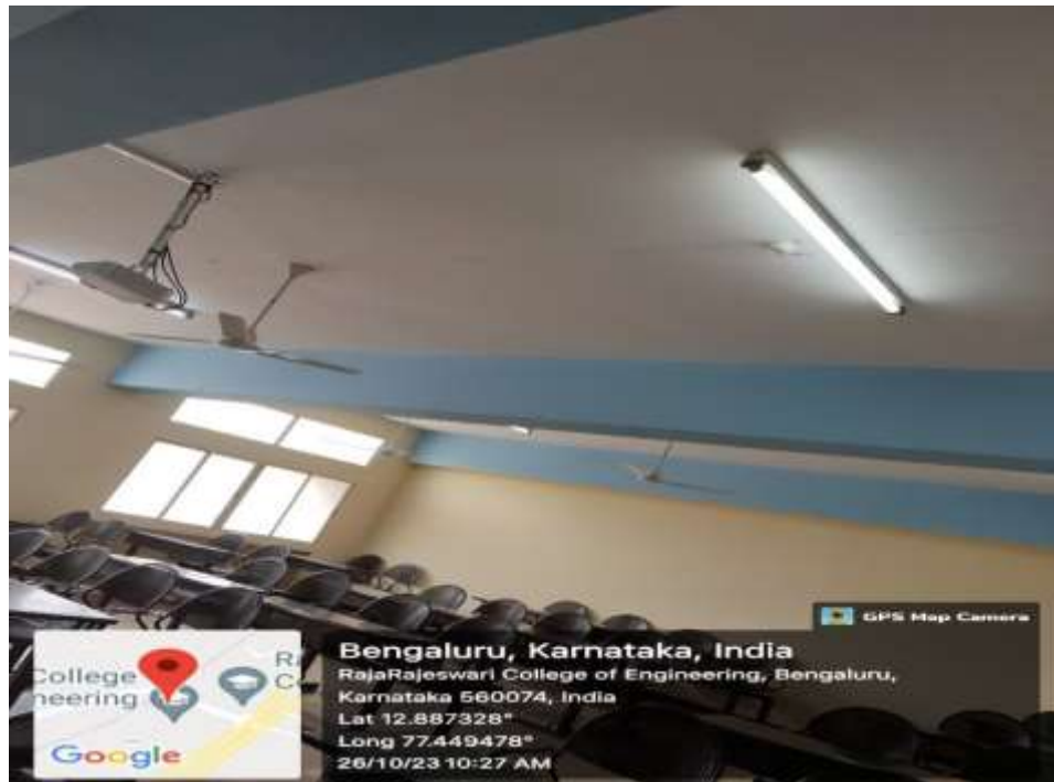
Photo.7: LED Tube lights in Classrooms at Rajarajeswari College of Engineering
