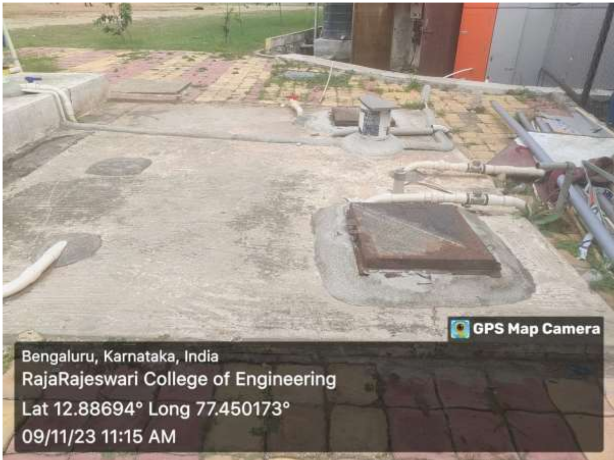
Photo.3: Water storage tanks in the campus
