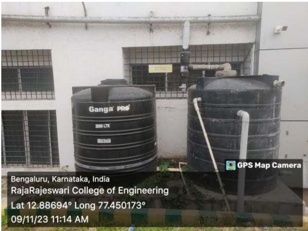
Photo.1: Rain water harvesting facility inside the campus
